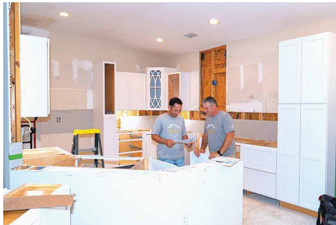
The full kitchen remodel at the Stine’s residence included new cabinetry & appliances, as well as electrical, plumbing and framing modifications to reach their vision. “They’ve done almost everything in our house, “I would absolutely 100 percent recommend them without any reservations at all,” says homeowner Idame Stine.
